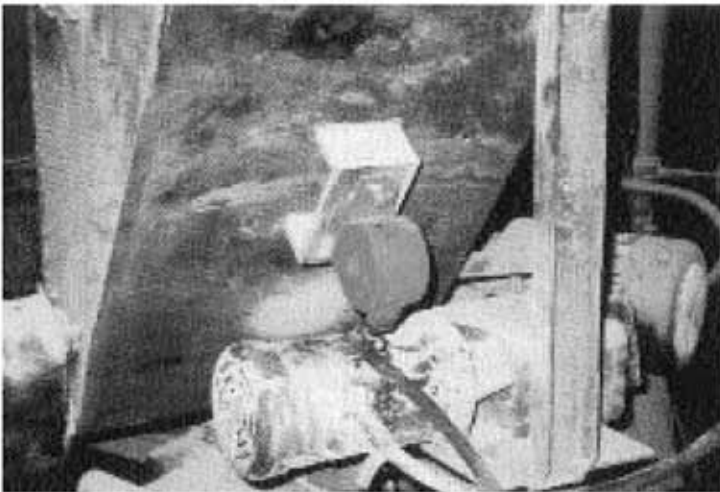
SILENT Turbine mounted to a fly ash chute to keep ash flowing.
